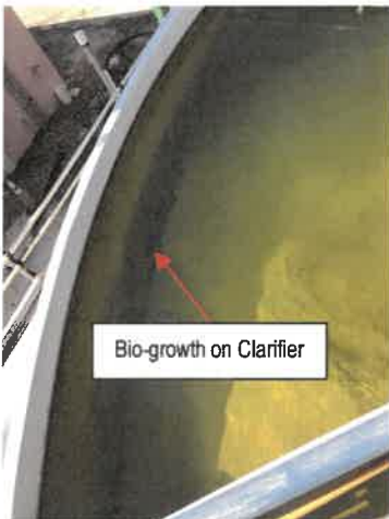
Picture 3: Bio-growth on Clarifiers
