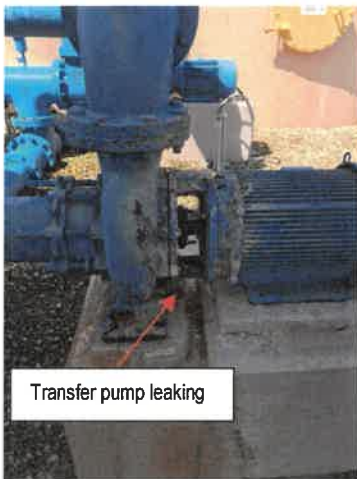
Picture 1: Leaking Transfer Pump
