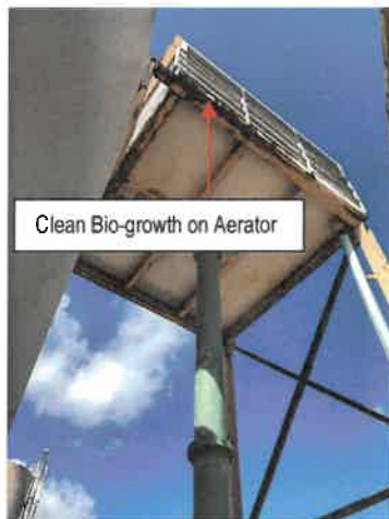
Picture 4: Bio-growth on Aerator
