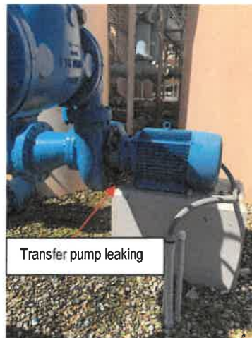
Picture 2: Leaking Transfer Pump
